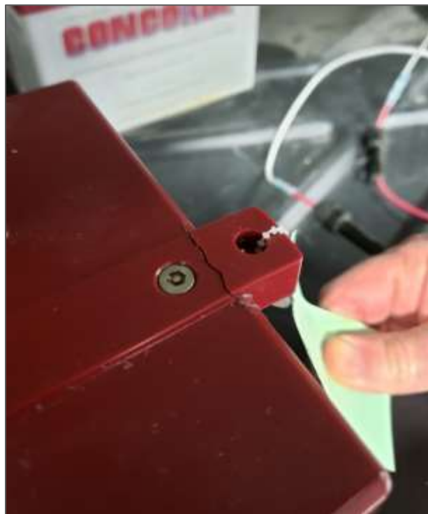
Figure 1. Cracked battery mounting tab
