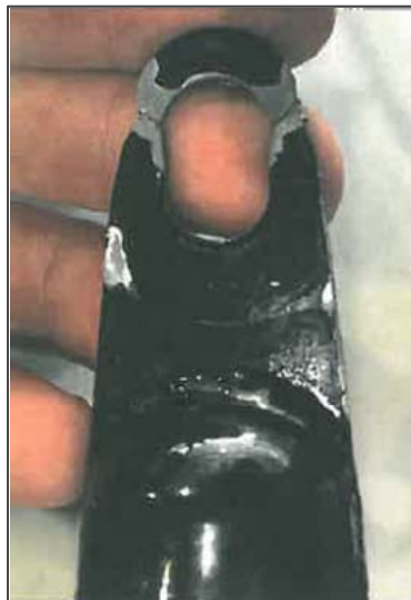
Figure 1. Failed drag strut attachment plate
