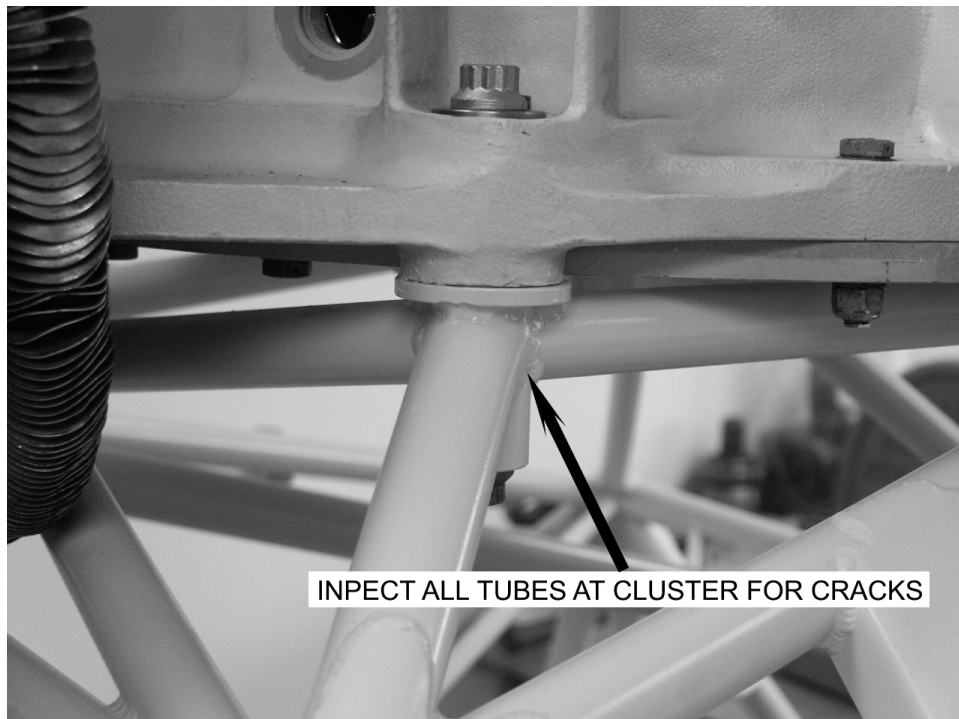
Figure 4. Right, Rear Main Rotor Transmission Mount Cluster
