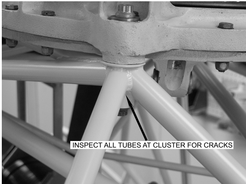
Figure 1. Right, Front Main Rotor Transmission Mount Cluster
