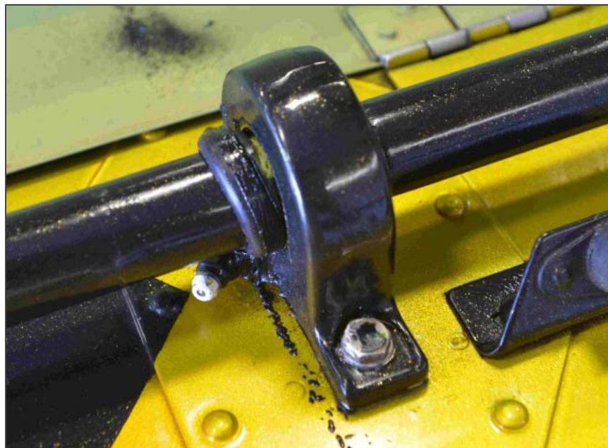
Figure 1. Bushing Deterioration (forward side shown)
